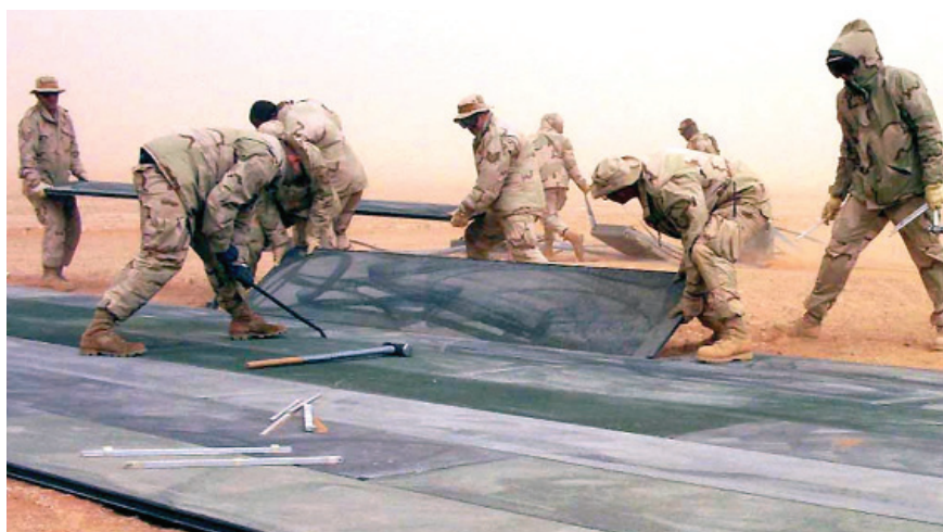
Temporary runway: – Deployed airmen of the 447th Air Expeditionary Group lay a portion of a temporary runway at a forward-deployed location during a driving wind storm. The group's job is to provide a place from which warfighters can operate. PHOTO: USAF
